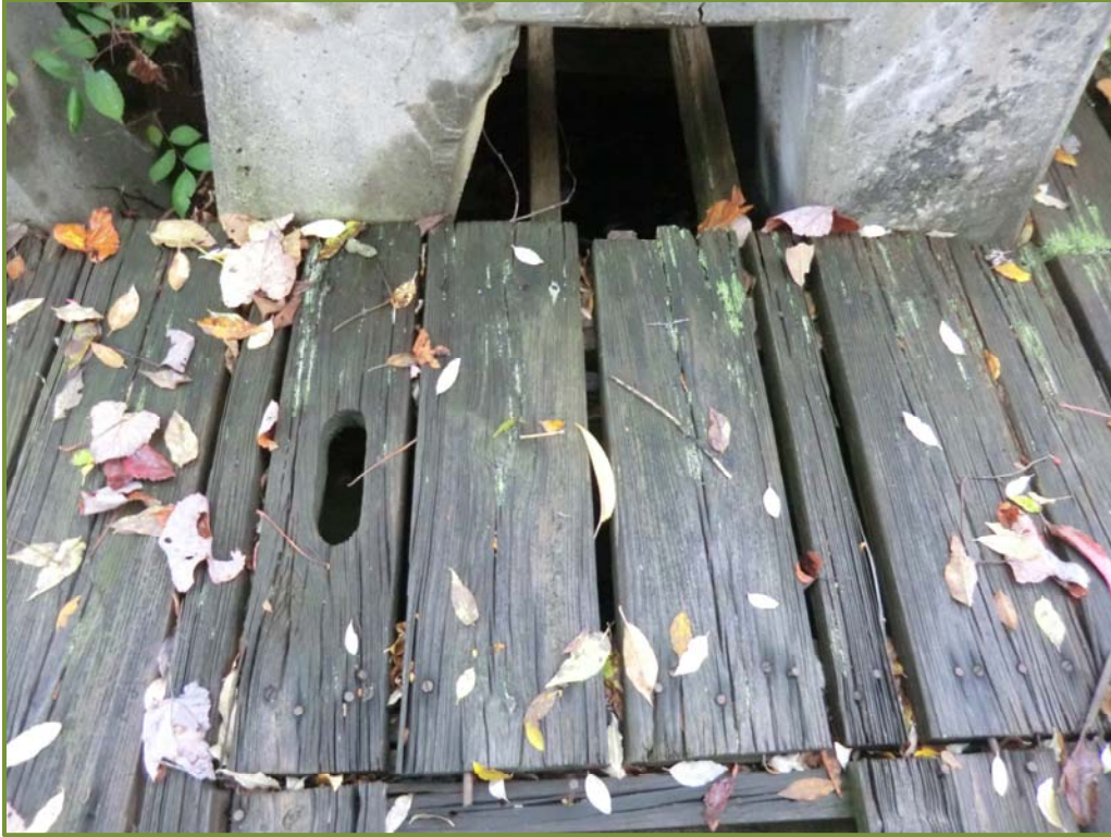
Photo 9. Detail of closed trap door leading to base of 5-m pillar, looking southeast
