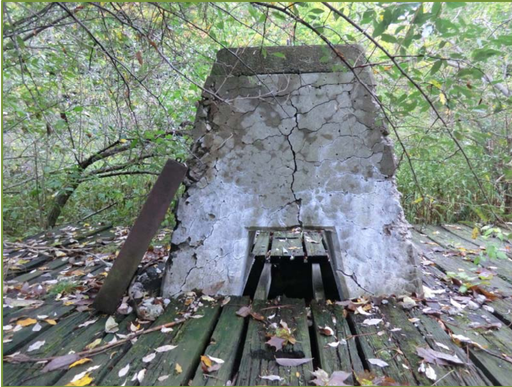
Photo 15. 125-m pillar showing cracking, looking southeast
